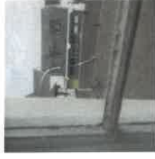
Front room window - replace damaged glazing
