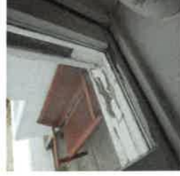
Rear ground floor windows – example of requirement to repair cill and frame requirement to repair cill and frame
